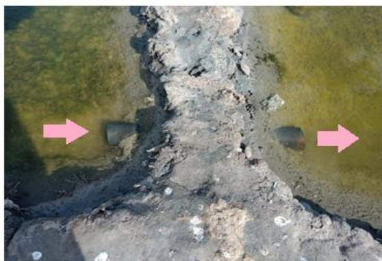
Figure 3. Seawater flowing from one compartment to another (arrow) through the PVC pipe.
